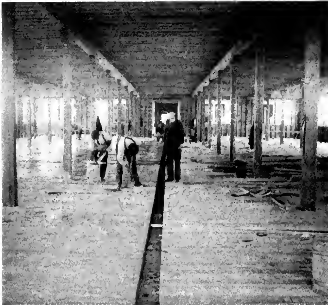
Interior view showing frame construction and wood floor. Floors are double with slushing between.
